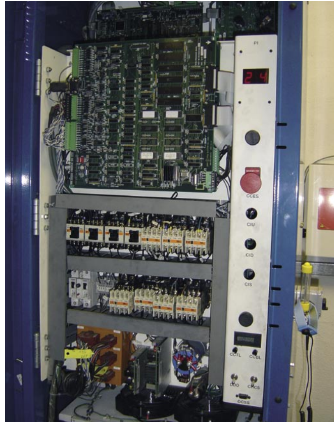
The existing Otis equipment.
