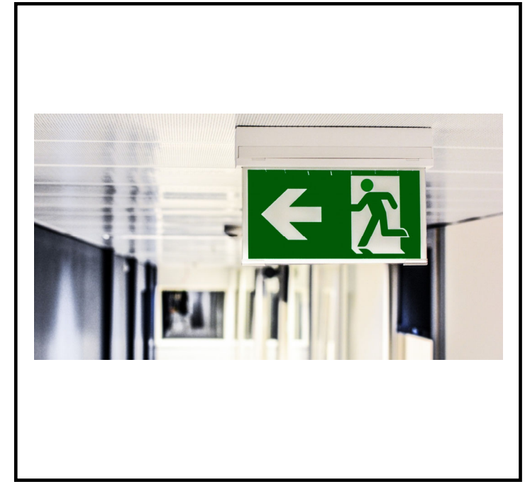
Designated fire escape routes
