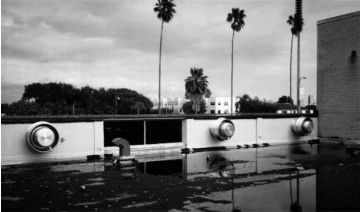
ASHRAE info: Photo #3 Side wall exhaust fans on apparatus room exterior wall, located above living quarters roof.
