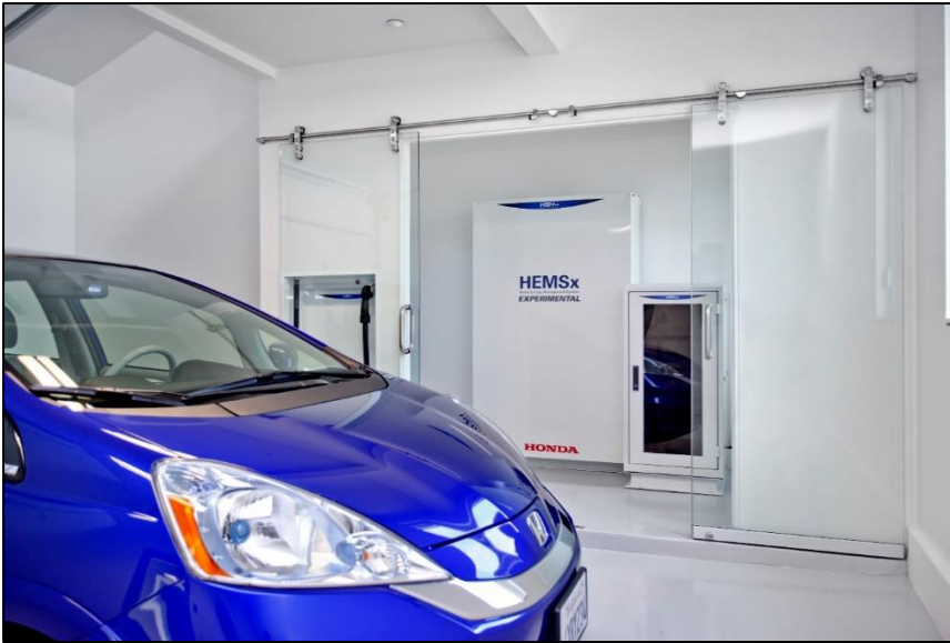
Figure 9 HEMS system in the garage with Honda Fit EV
