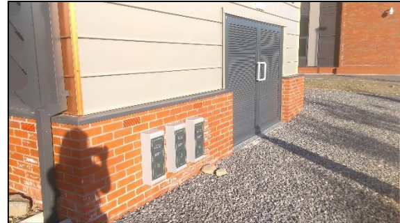
Figure 17 Charging points at the Active Office
