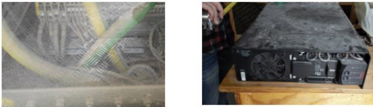
Dust over cable and UPS
