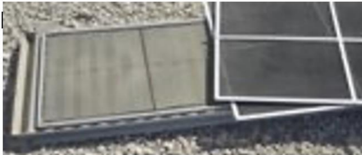
Dust jamming the ventilation filter in comparison
