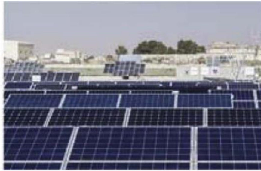
Solar PV farm(250kW)
