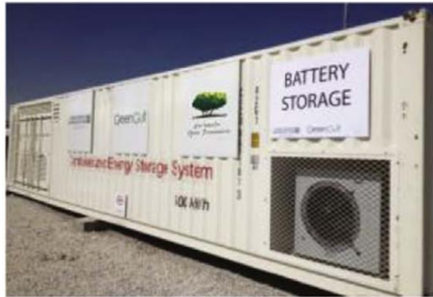
Battery Storage System(250kW/500kWh)
