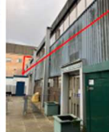
Photo 13: DH primary pipework to be supported at mid level by primary steel members
