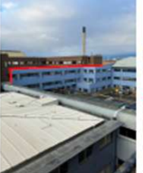
Photo 11: DH primary pipework runs at HL above 4A walkway.
