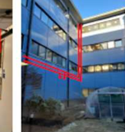
Photo 17: DH primary pipework routes across the lower courtyard facade to enter plant rooms AFB_00_VENT and AFB_00_WATER. Pipework to AFB_00_WATER will also need to be routed through the internal corridor.
