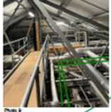
Photo 9: DH primary pipework to be distributed in the BR ceiling void. Pipework to be complete with drip trays where above critical spaces.
