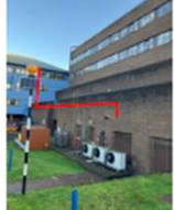
Photo 10: DH primary leaves roof void, drops and enters 4A plant-room at HL.
