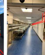
Photo 16: DH primary pipework to be housed in basement/corridor connecting buildings BR and 4F.
