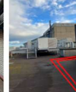
Photo 15: DH primary pipework to be installed using "big foot" system or equal and approved. Pipework to route across the roof and enter the OPD_ROOF at high level.
