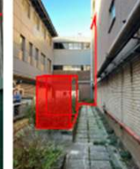
Photo 14: DH primary pipework drops down, crosses brick facade and enters new external plant space housing DH equipment. Step overs to be provided for low level services.
