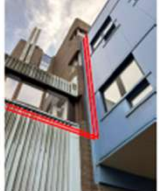
Photo 12: DH primary pipework drops in corner and turns to run just below windows.
