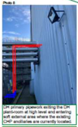
Photo 8: DH primary pipework exiting the DH plant-room at high level and entering soft external area where the existing CHP excavations are currently located.
